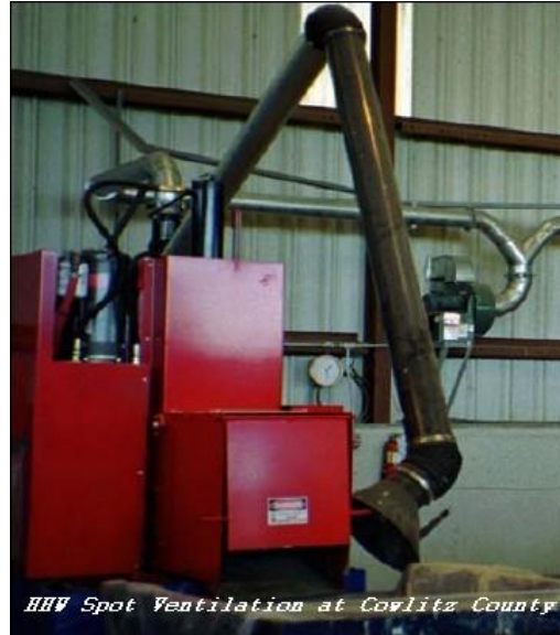
Local Ventilation connected to Hepa Filter
